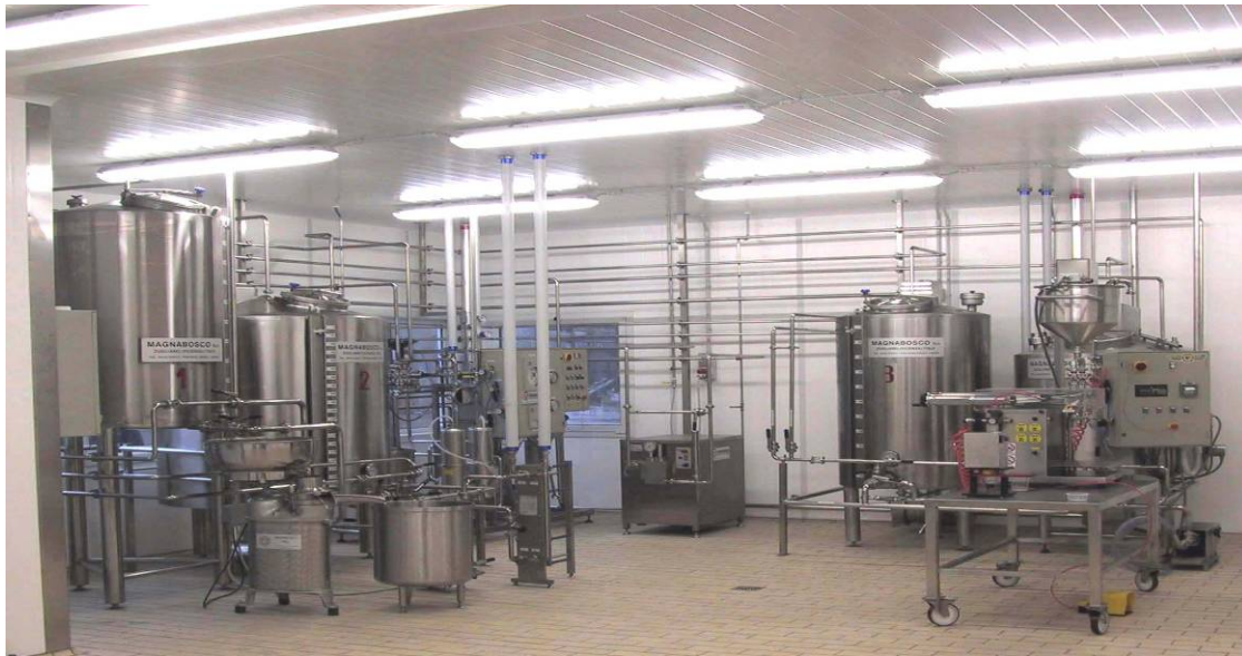
The whole plant
