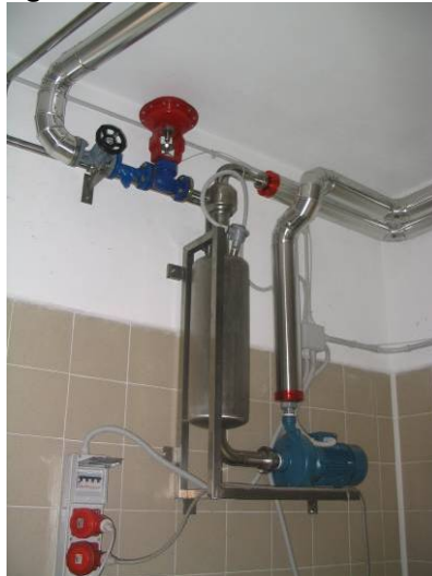
Hot water line
