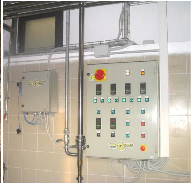
Milk receiving tanks running panel
